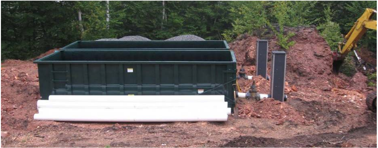
Photo 7. Mitchell Roll Off systems under construction. The West Box is in the foreground with the East Box behind. The 8" valves and Agri Drain smart drainage systems have been installed.
