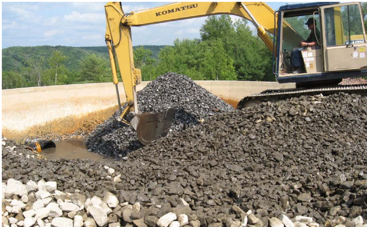
Photo 20. Mitchell Tank limestone cleaning. Standing water sump used to mechanically wash stone. Black pipe is effluent pipe carrying solids out of the system to the settling pond.
