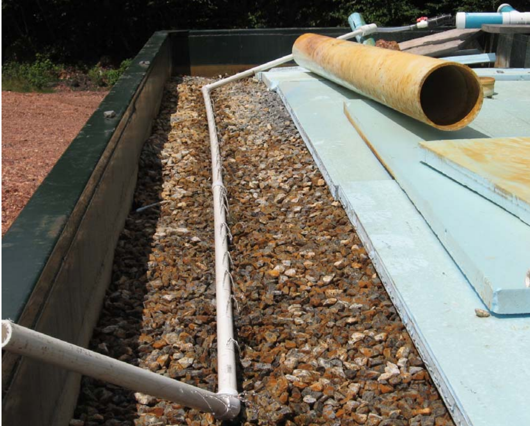
Photo 25. Flow distribution system installed in West Box.
