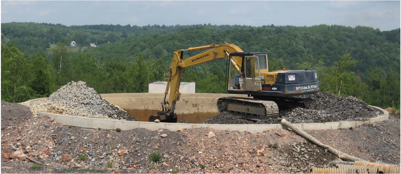
Photo 19. Mitchell Tank limestone cleaning. Cleaned limestone is visible in the left side of the tank. The excavator is sitting on top of limestone that has not yet been cleaned.
