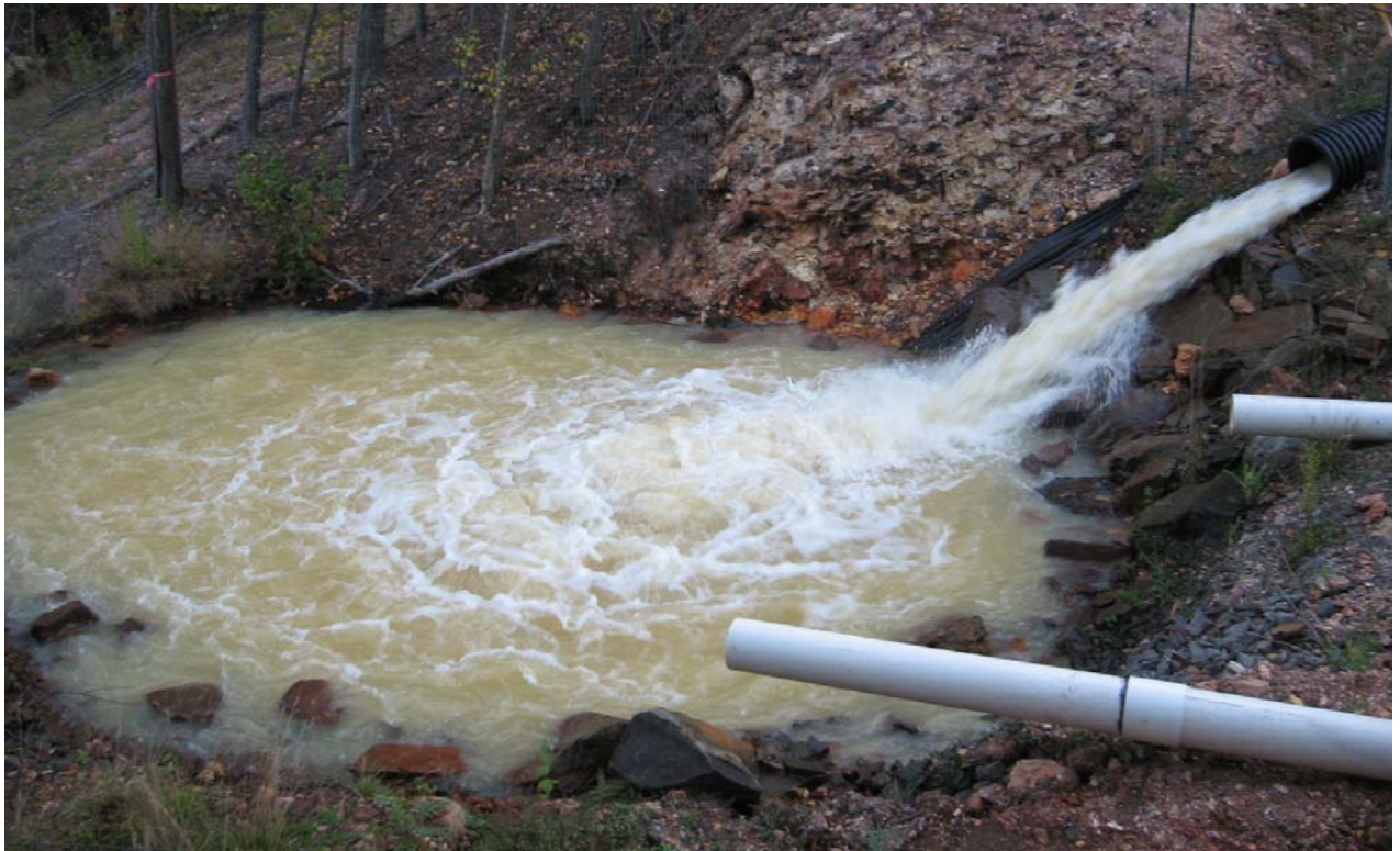
Photo 5. Mitchell Tank flushing into energy dissipater.
