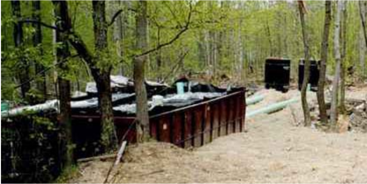
Photo 1. Jonathan Run systems before insulation was installed. The roll off container on the right is Box 1 and Box 3 is on the left. The siphon vaults are visible to the right of the roll off containers.
